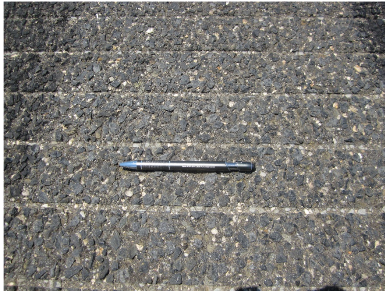
Figure 19. Example of severely eroded grooved surface.
