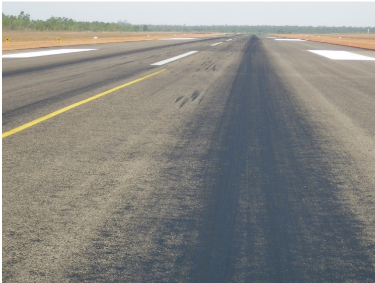
Figure 13. Example of wheel path flushing of a sprayed seal.
