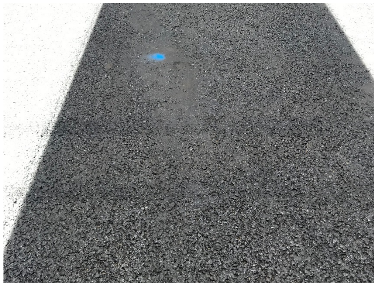
Figure 14. Example of isolated asphalt bleeding in SMA.
